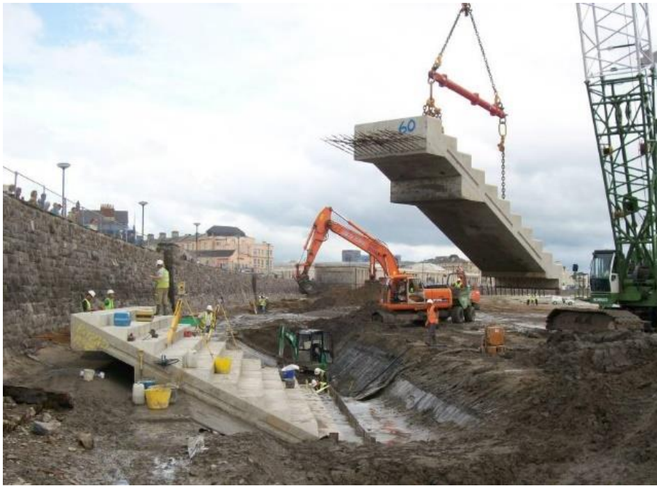
Images 3 and 4. At Weston-super-Mare, the Victorian sea walls have already had an upgrade. Concrete steps have been built in front of the old walls to prevent waves from damaging the bottom of the wall. New walls were also constructed behind the promenade to protect properties from large waves that overtop the old walls. These were also designed so that they can be raised when needed in the future due to sea level rise.
